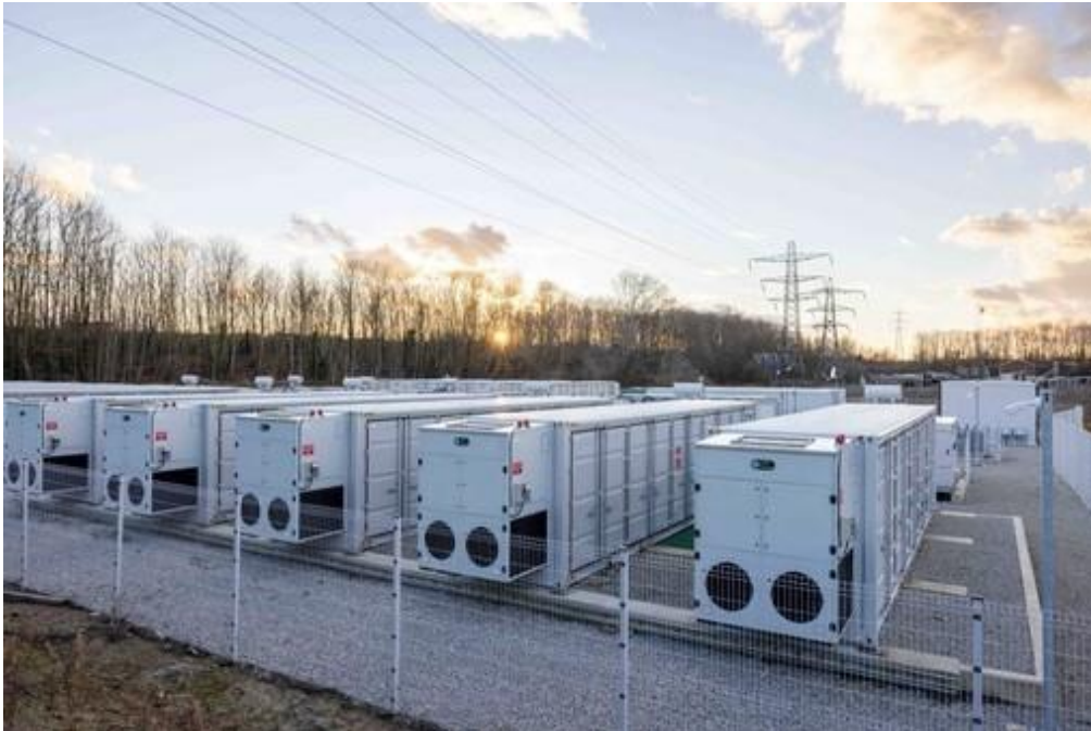
Figure 3-4: Example of a BESS Facility
