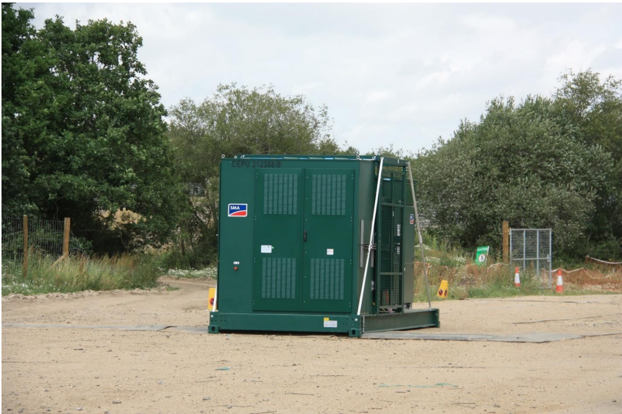
Figure 3-3: Example of a Central Inverter Container
