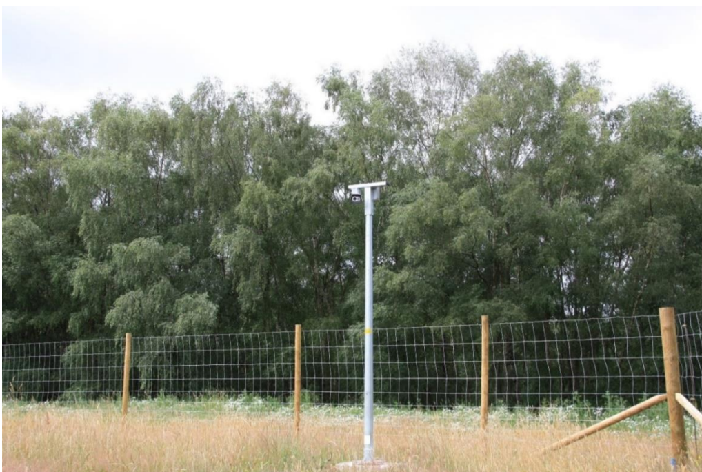
Figure 3-5: Example of Pole Mounted CCTV
