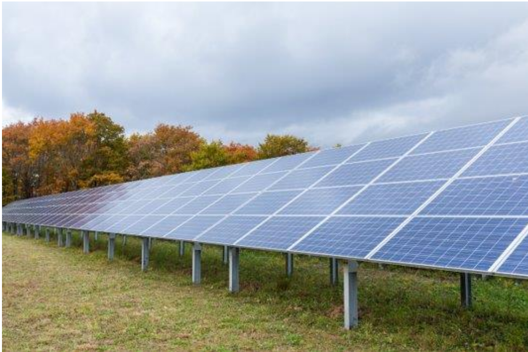
Figure 3-1: Example of a Solar Array
